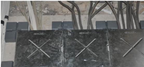
Management of old power and data cables
